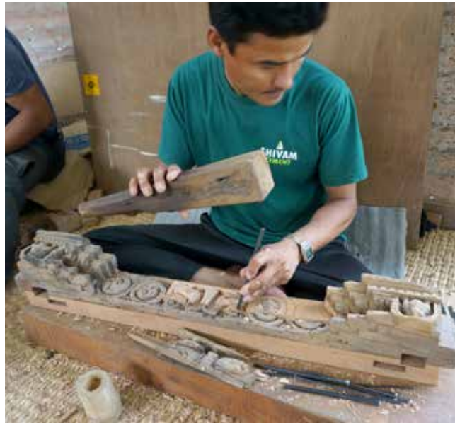
Char Narayan Temple | May 29 & June 03, 2016 Damaged part of the door pillar is replaced with a new wood where detailed carving will be done to match the original. Details of the carving are being added to the repaired and retrofitted door seal by a woodcarver.
