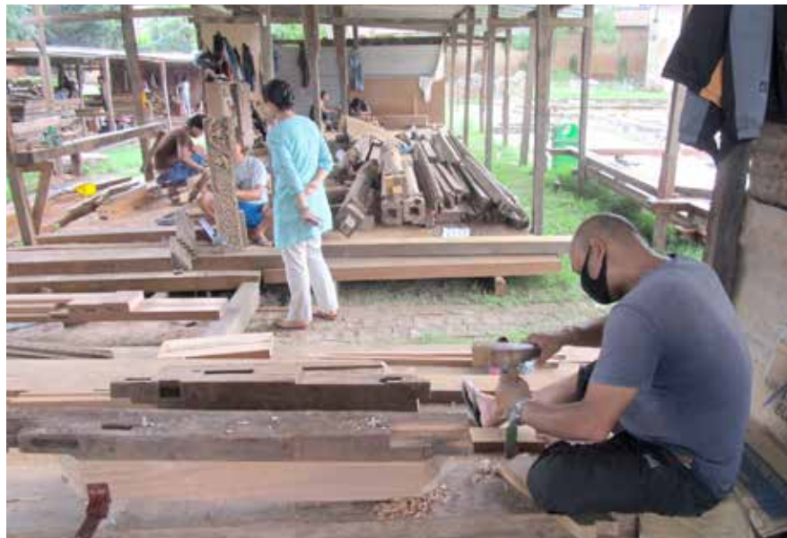
Char Narayan Temple | June 19, 2016 A view of workshop at Bhandarkhal Garden where woodcarvers and carpenters are repairing and replicating the damaged and missing parts of the doors.
