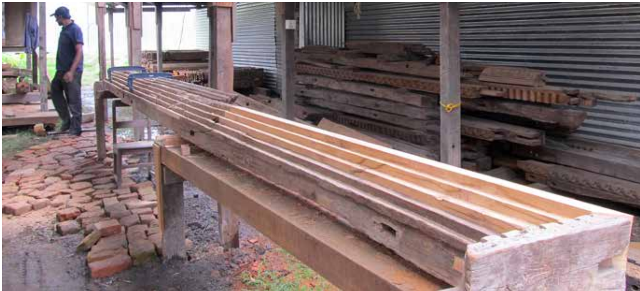
Char Narayan Temple | June 12 & 16, 2016 A part of the door during repair and after completely repaired.
