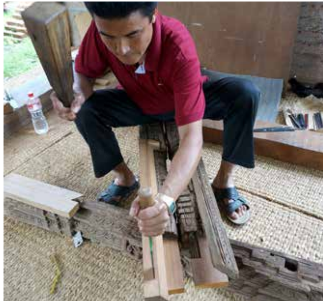
Char Narayan Temple | June 05 & 08, 2016 Damaged part of the door is being replaced with a new wood piece for replicating carving details and woodcarver replicating on it.
