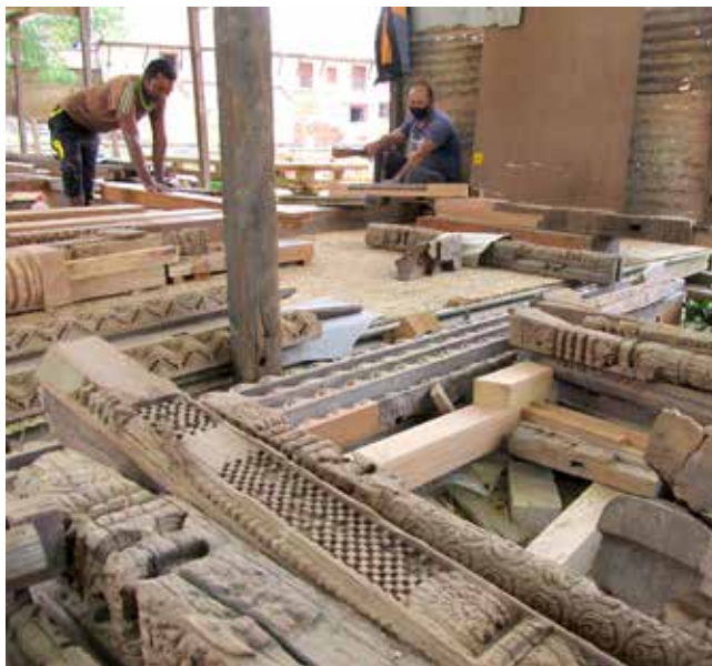
Char Narayan Temple | May 24 & 26, 2016 Doorframe is being repaired and retrofitted by replacing the damaged parts of the doors at the workshop.
