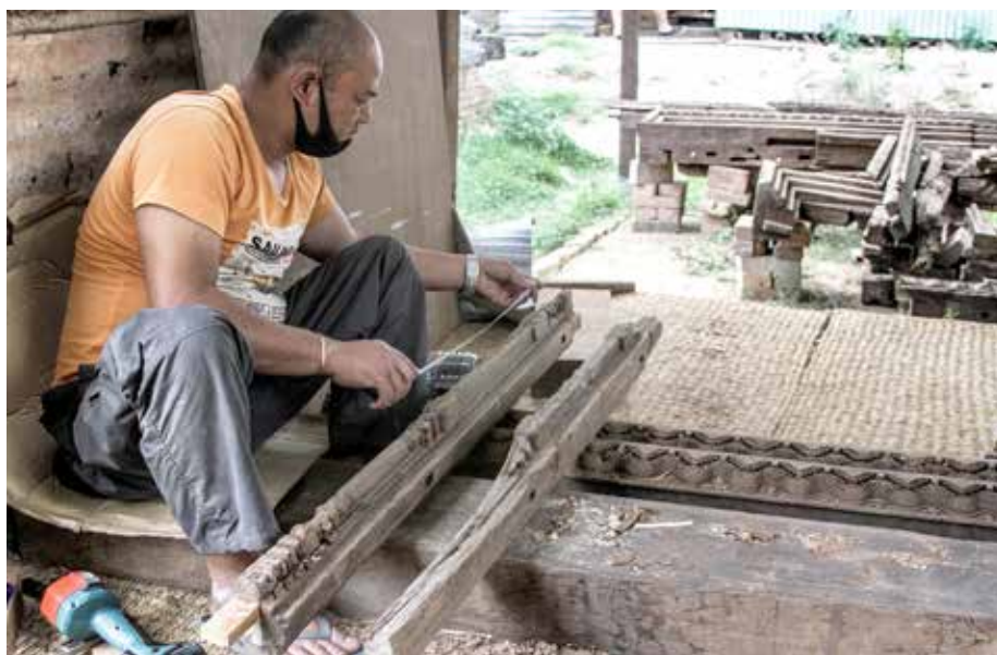
Char Narayan Temple | May 13, 2016 Carpenter/woodcarver Shyam Prasad repairing outer frame of one of the main doors.
