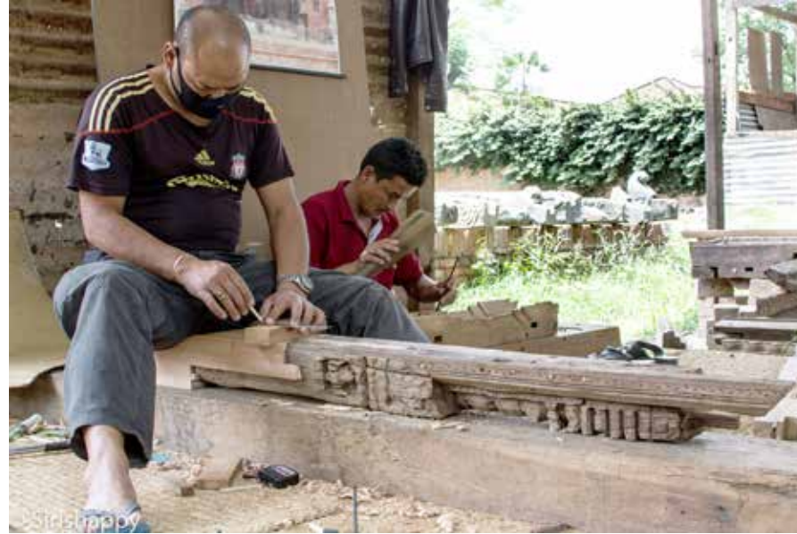
Char Narayan Temple | May 17, 2016 Woodcarver prepares plain timber part of the window for the carving. Woodcarver Shyam Prasad Silpakar replacing the damaged section of south facade doorframe.
