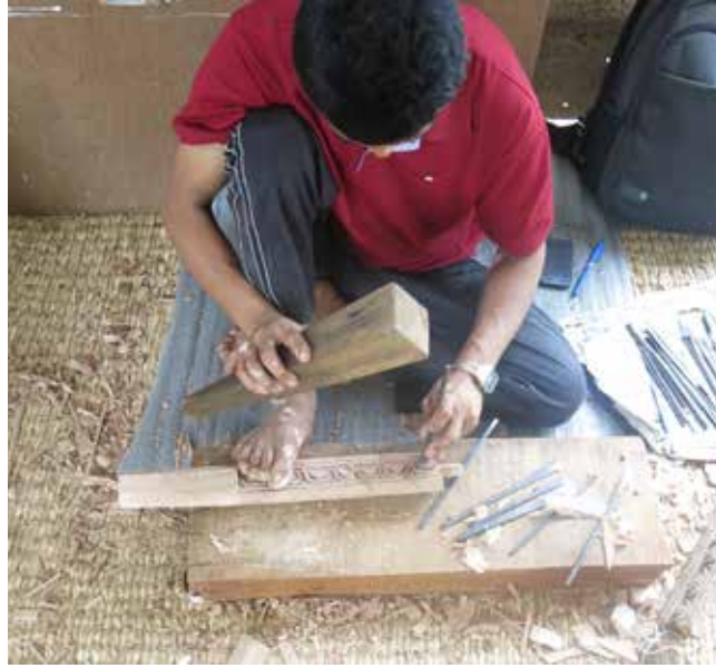
Char Narayan Temple | May 05, 2016 One of facade door is being inspected for repair and retrofitting work. Woodcarver replicating the missing kulah (cornice) of the door.
