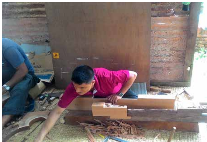
Char Narayan Temple | June 21, 2016 Woodcarver adding details of existing door parts to the new timber piece.
