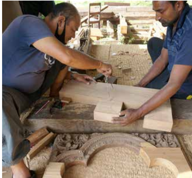
Char Narayan Temple | June 05 & 08, 2016 The arch of the main door is being repaired by adding new piece of wood for replicating carving details.
