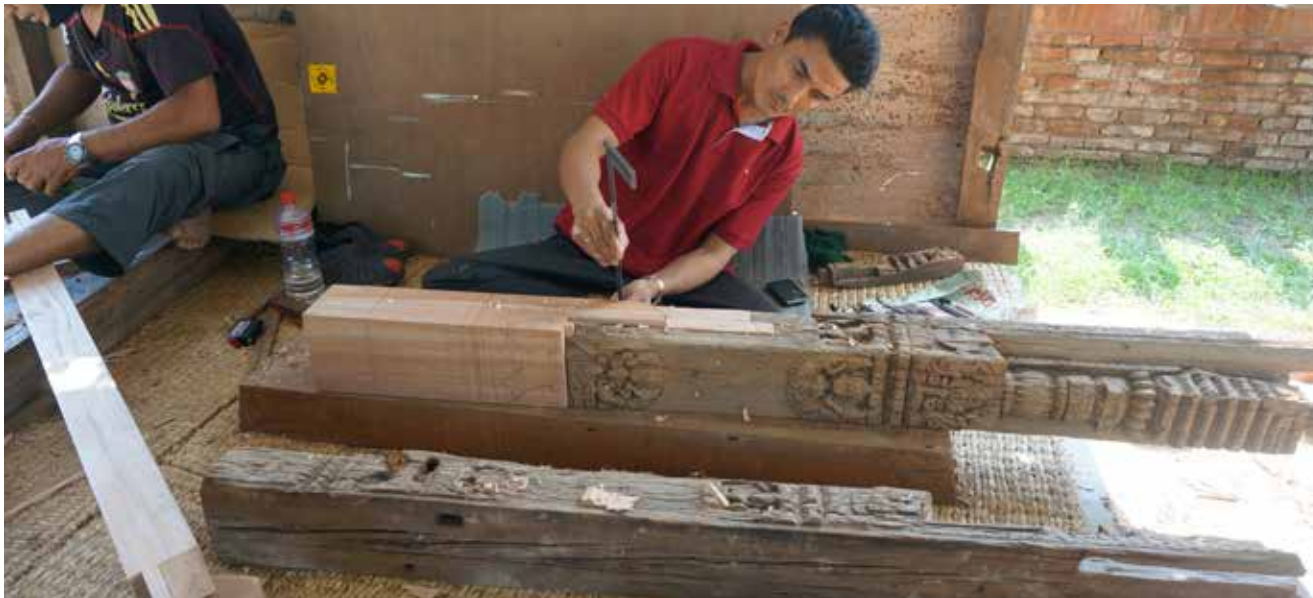
Char Narayan Temple | May 20, 2016 Doorframe is being repaired and retrofitted by replacing the bottom part of the column.
