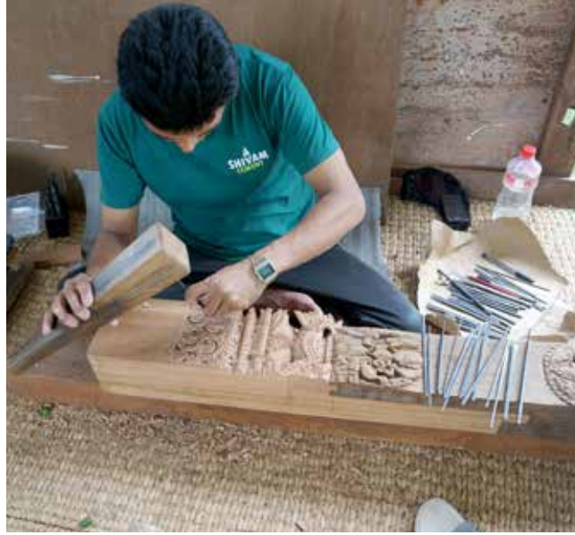
Char Narayan Temple | May 30 & June 01, 2016 Door jamb ( mubaha ) after addition of new timber and during carving replication.
